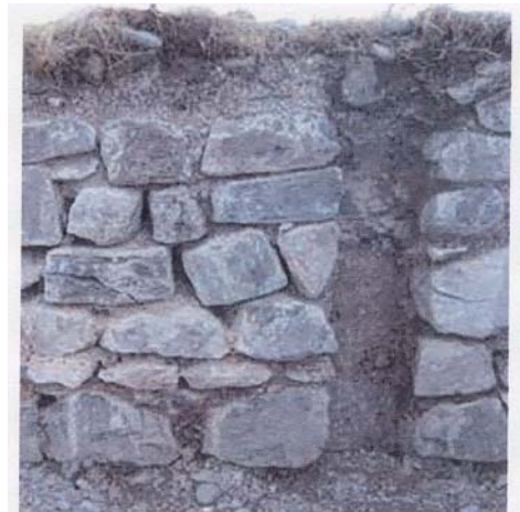
The curtain wall, the gap was formed by a decayed 'nailer post' . (CBC Photo / Jenna MacNeil)
